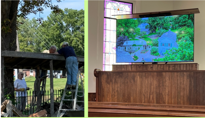
Left: Volunteer Jim looks up as volunteers Lynn and Jeff install new shingles on the wood stack lean-to behind the cabin. Right: Our new audio-visual set up sits on top of our beautifully built AV cabinet!
