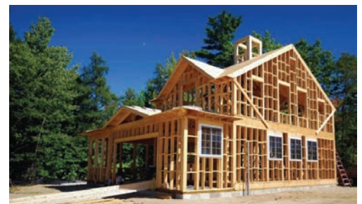
The Village's General Store is a modern structure built in 1989 to represent the general store that was located at Troy Corners. The City of Troy utilized modern platform framing techniques as seen in this image for our structure
