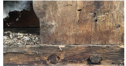
Recent preservation work on the Caswell House enabled us to get a peek into its timber framing. Here you can see corner bracing and the mortise-tenon-peg joints utilized in this building technique.
